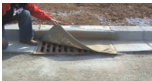
Inlet protection on a storm drain.
