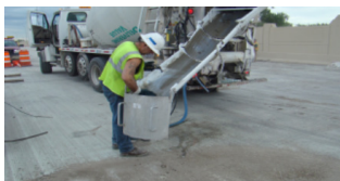
Chute washout system.
