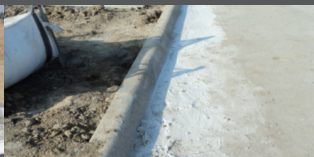
Illegal discharge to storm sewer!
